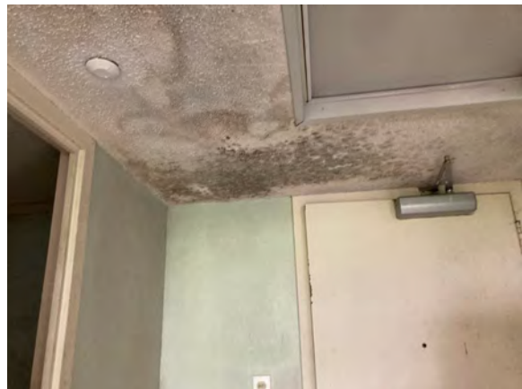
Photo of ACM Ceiling Texture (off-white) on 3 rd Fl.
