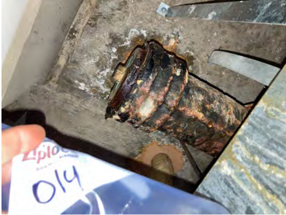
LTBA-006-PLM-014 Pipe Mastic (black) above drop ceiling in Lobby.
